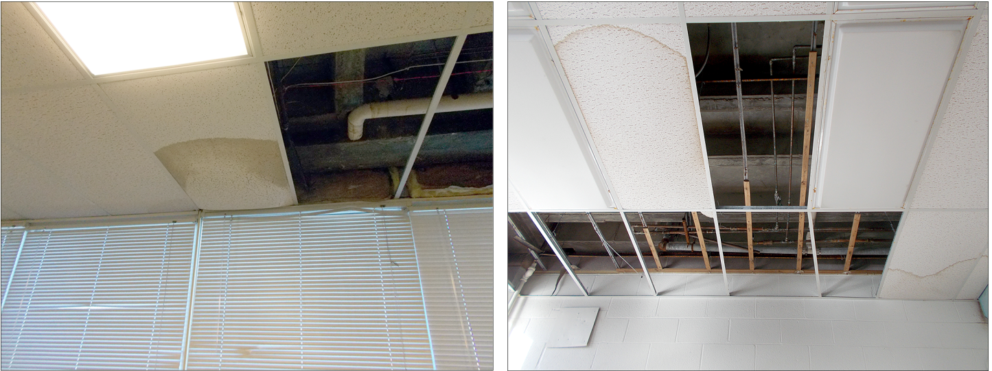
Figure 4: Damaged or Removed Classroom Ceiling Tiles Due to Leaks in Recently-Installed Roofs
