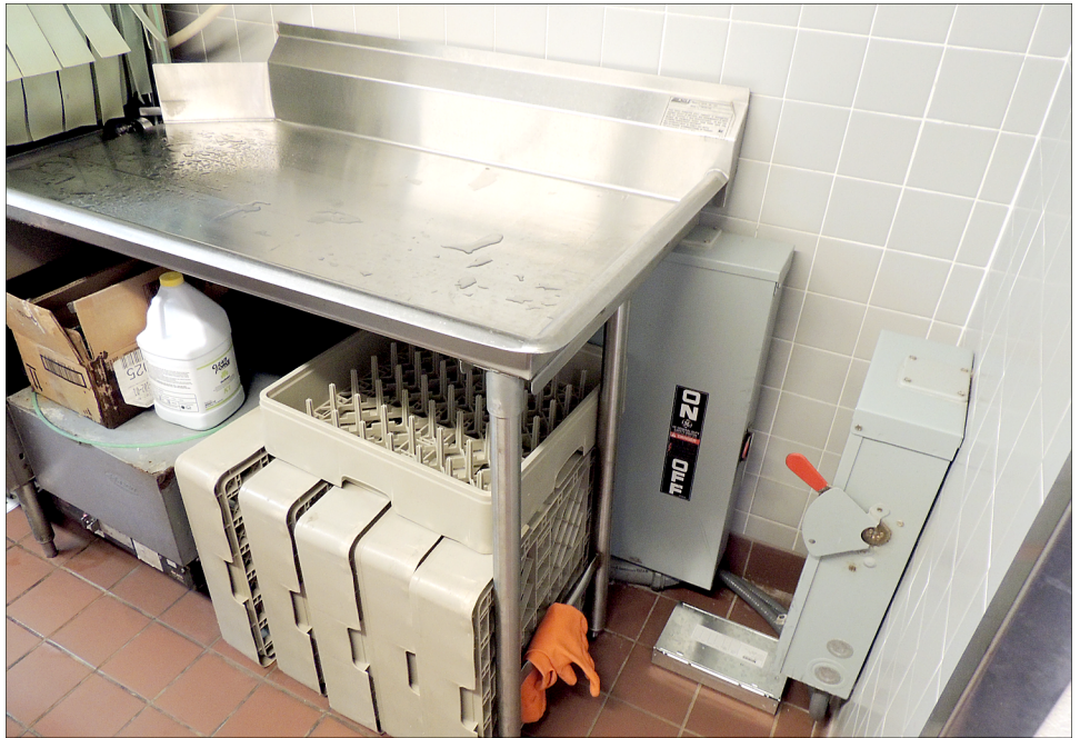
Figure 5: High Voltage Electrical Panel Installed Next to Cafeteria Dishwasher at a BIE-Operated School, October 2014
